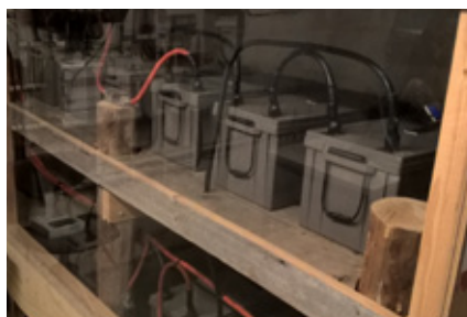
As energy production and use at the site may fluctuate greatly at different times, the battery balances the difference between the production and generation of power.
